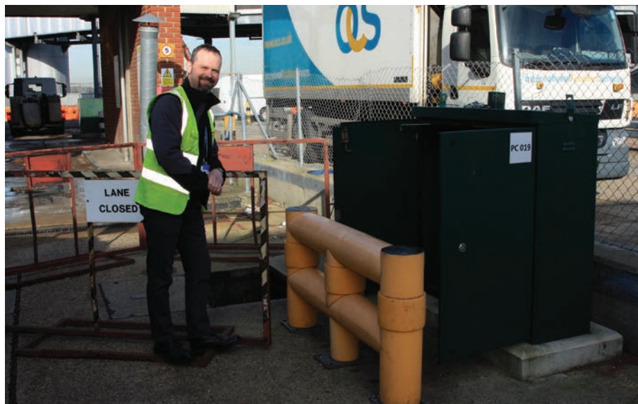
Below. Ian Jolly, system specialist for water services at Heathrow Airport, works with the Flygt Concertor during the system trial.
